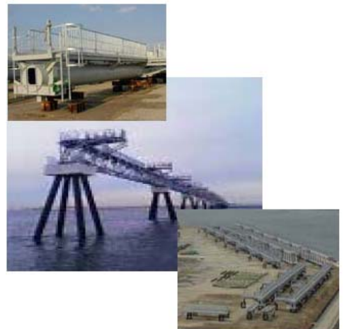
HS-100 PERMEATE was used on the landing approach light apparatus built in the ocean at the Kobe International Airport in Japan
